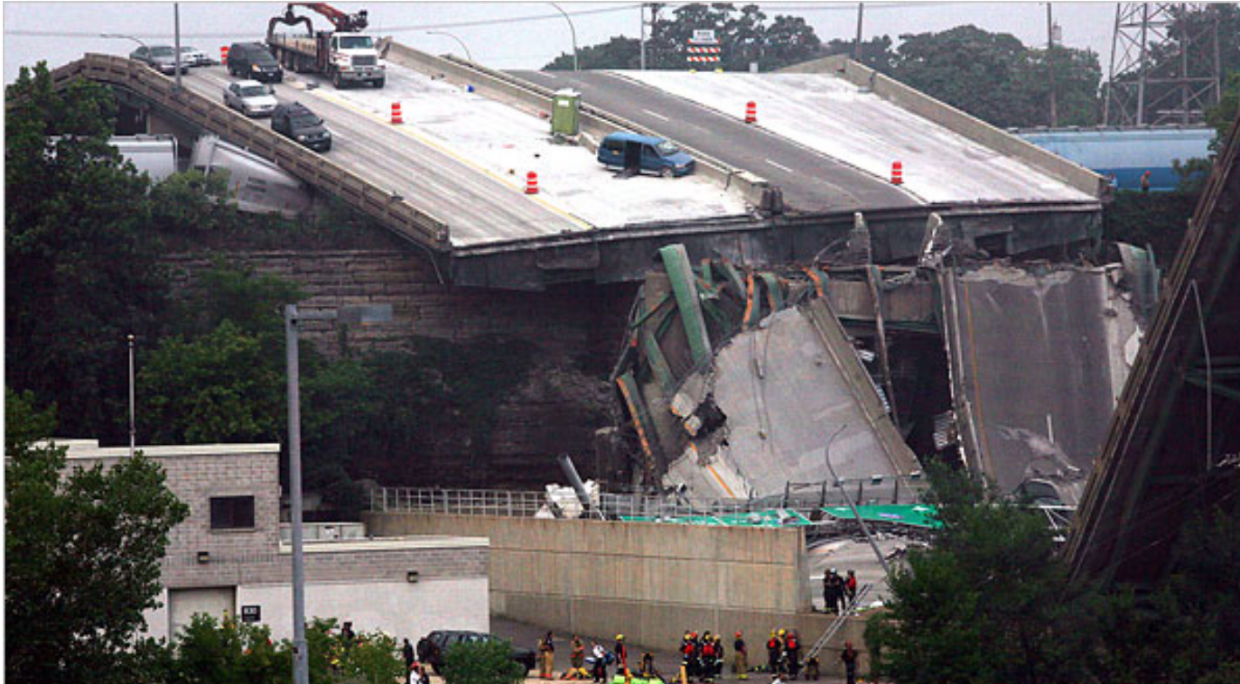
Collapsed I35 W. Mississippi Bridge, August 1, 2007.
